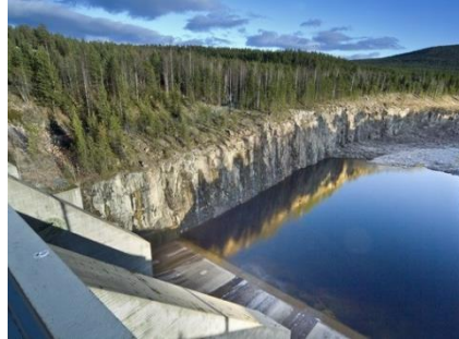
Power Generation – Generation
