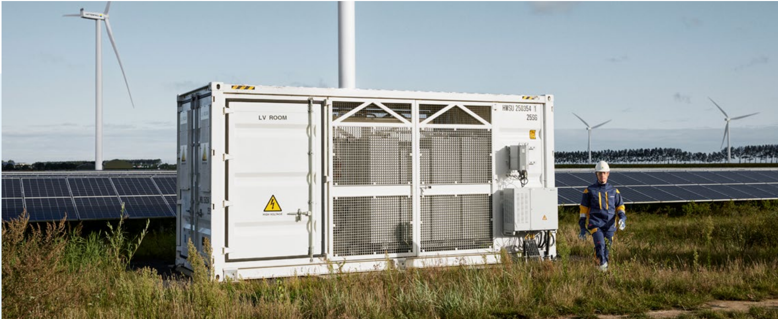
Solar and batteries 10.9 GW of solar and battery capacity in development², including the 254 MW Brunsbüttel Battery Project in Germany. ² including capacity managed but not owned
