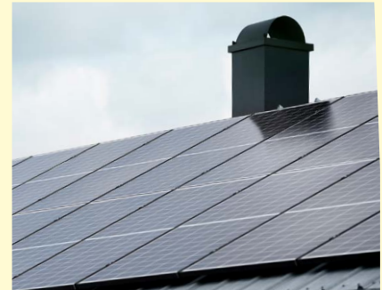
Solar panels enable our customers to integrate decentralised fossil-free electricity.
