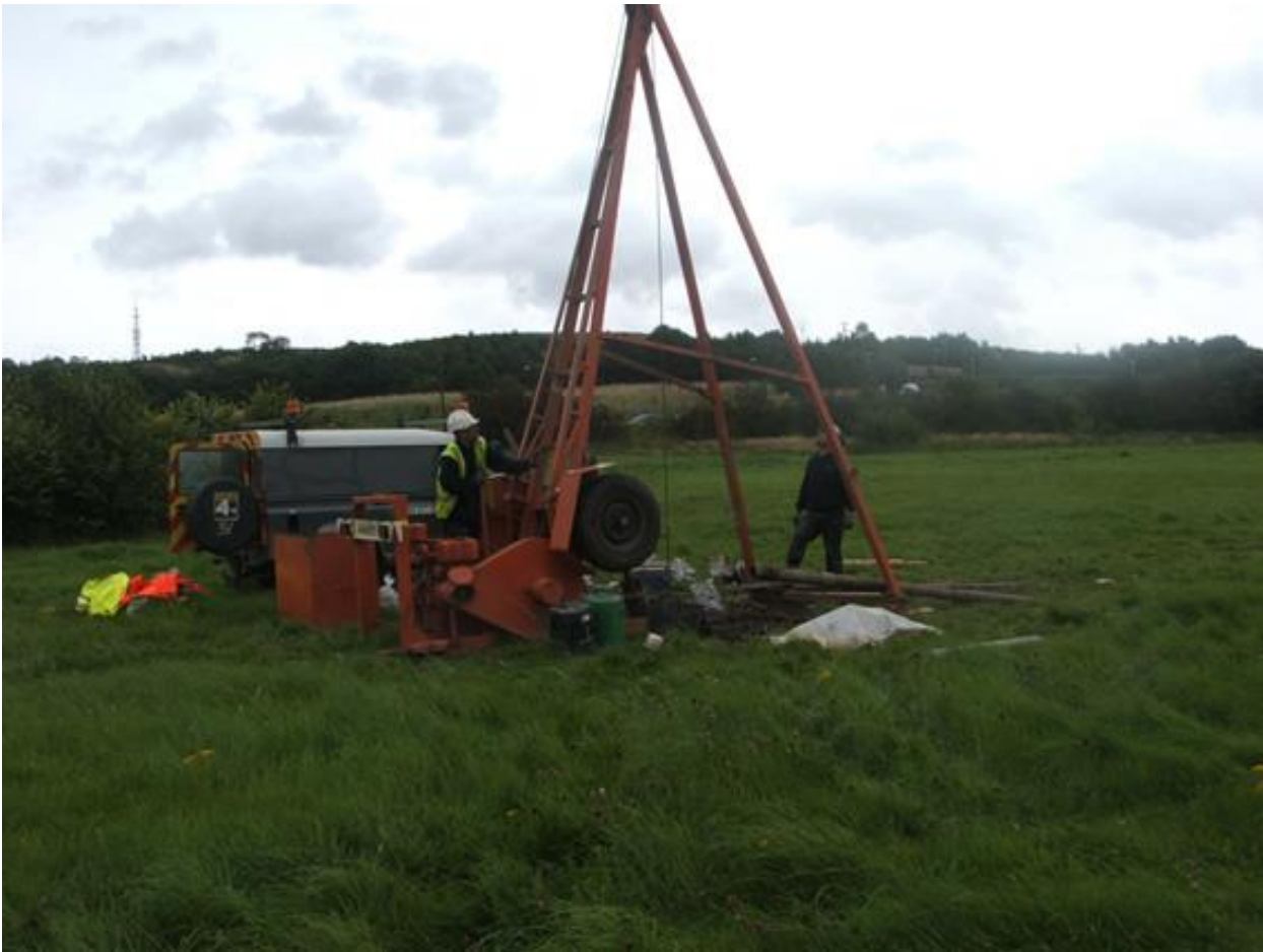
Fig 1. Picture of a borehole drill rig of the type that will be deployed locally.
