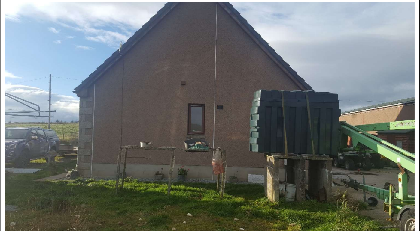
View of the east facing façade showing a single small frosted window
