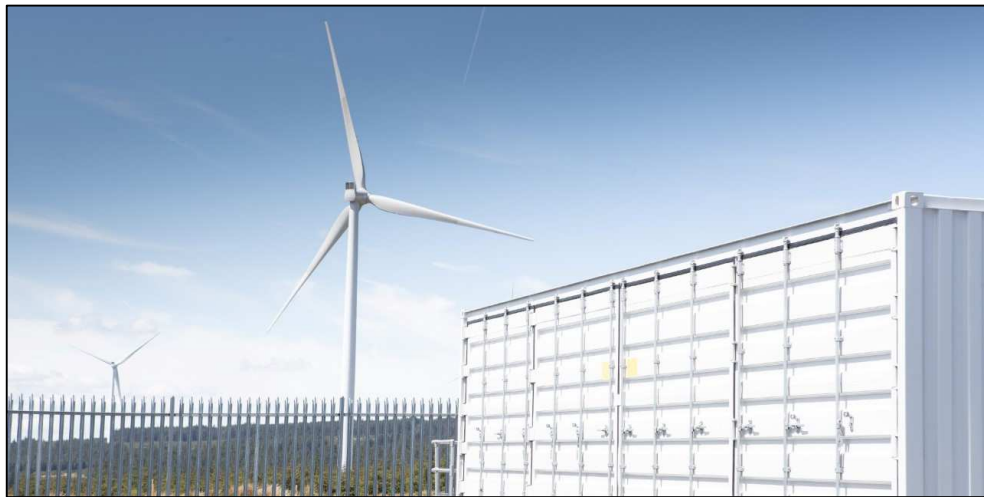
Plate 1: Battery storage units at Pen y Cymoedd
